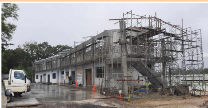
PROGRESSING TOWARDS COMPLETION: ROOF STEEL STRUCTURE INSTALLATION UNDERWAY AT THE CTC MULTI PURPOSE TECHNICAL BUILDING.
