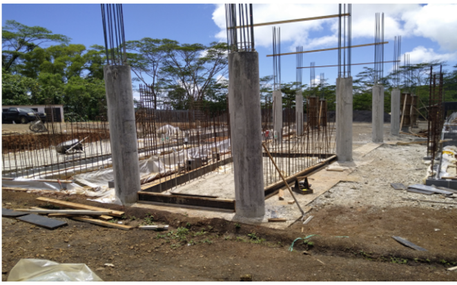
BUILDING THE FOUNDATION: COLUMNS AND FOUNDATION WALLS RISING TO THE FLOOR LINE AT THE NATIONAL CAMPUS STUDENT CENTER, CAPTURED FROM THE EAST END.
