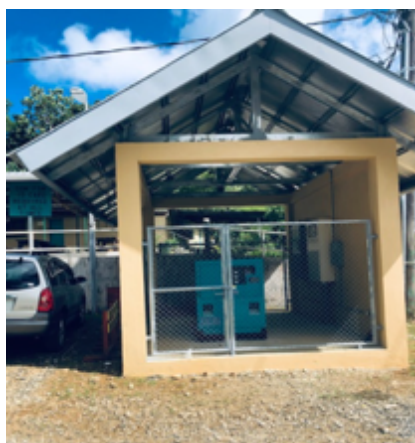
Career & Technical Education Center (CTEC) now has a backup generator installed so classes can continue during power outages.
